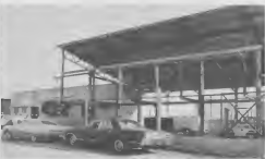
Granville Arrindell's shop and office addition is about four times his present shop space. The 2100 square foot new shop space and a 600 square foot second floor office will cost about Fls. 80,000.
